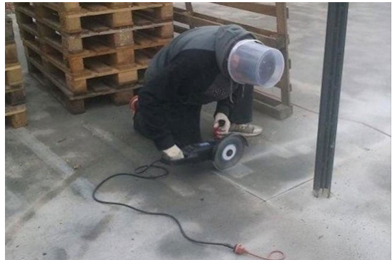
Is this hazardous?
