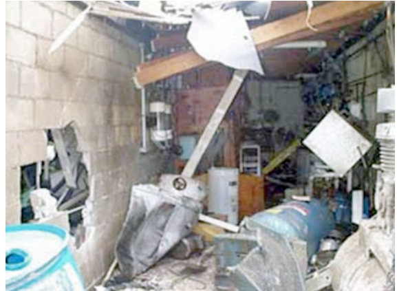
Air Compressor Explosion
