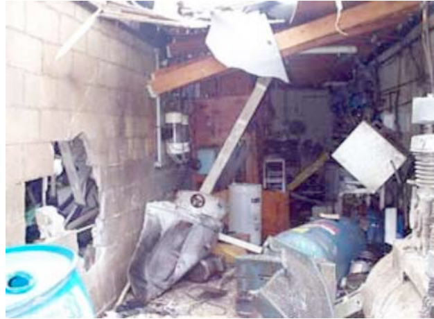
Air Compressor Explosion
