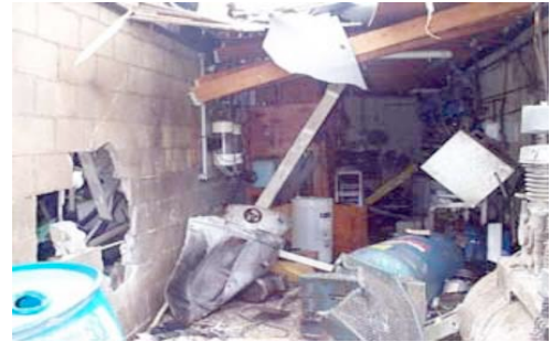
Air Compressor Explosion
