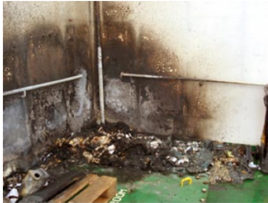
FIRE CAUSED BY SPONTANEOUS IGNITION (OILY RAGS)
